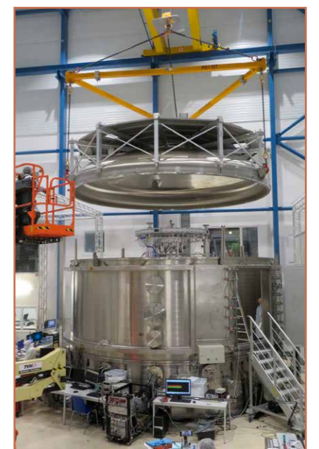
Installation of the SILENT prototype at PML.
