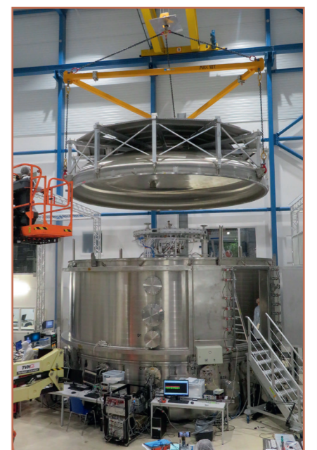
Installation of the SILENT prototype at PML.
